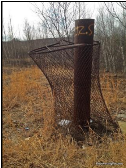
A smoke vent in Centralia
